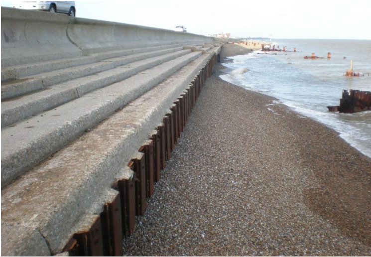
Exposed sheet pile toe at Slaughden, south of Aldeburgh – February 2015
