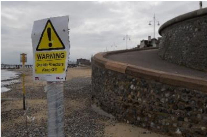
The failing Flag Pole Ramp
